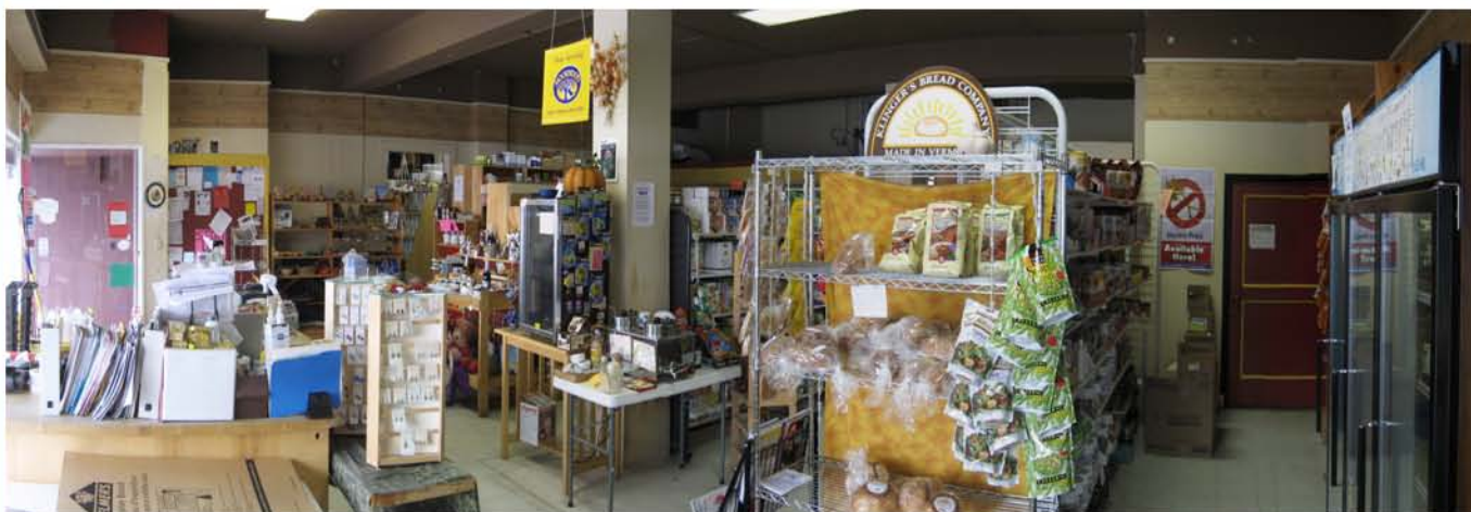
Before the Renovation — grimy floors, crowded floor space, faux wood wallpaper, and a brown ceiling in need of repairs.
